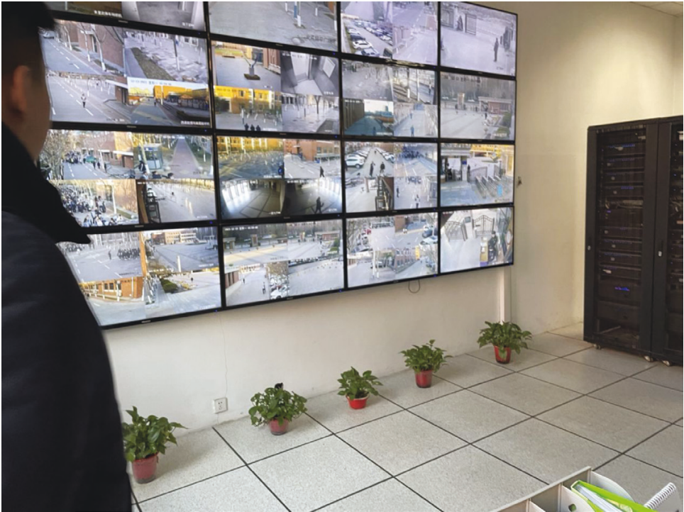
Fig. 7 The central control room at R School (photo taken by authors: November 2021).
