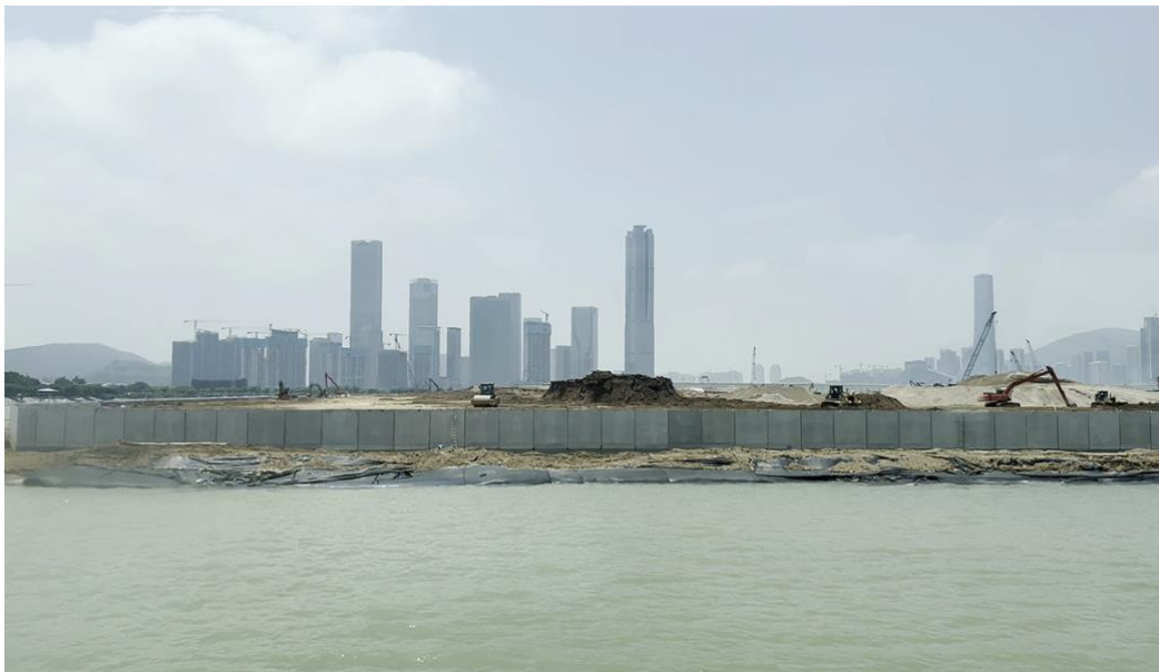
Land reclamation project in Macao New Urban Zone C (Photo by author, 2022).
