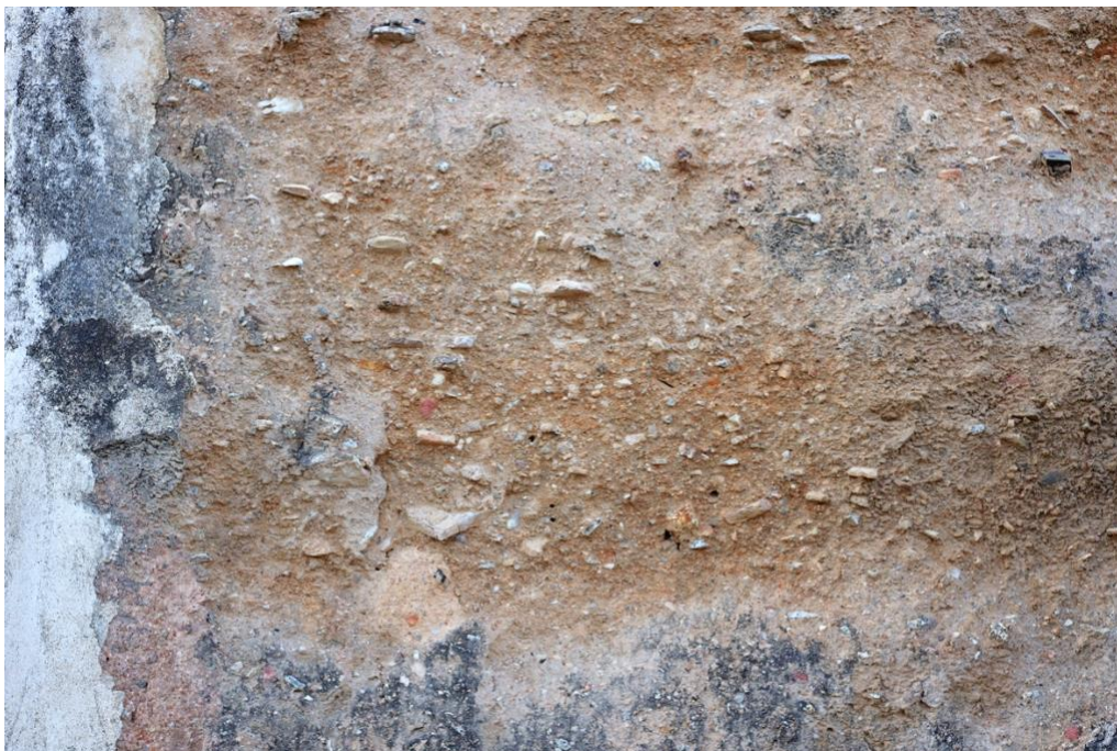
Section of city wall in Macao made of chunambo (Photo by author, 2022).
